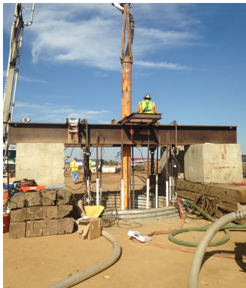
Construction has begun on California's high-speed rail system. Photo courtesy of the California High-Speed Rail Authority
